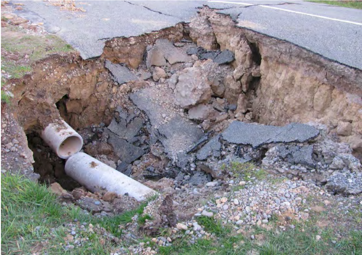
Figure 9 Damage to underground services as a result of liquefaction, Christchurch 2011.
