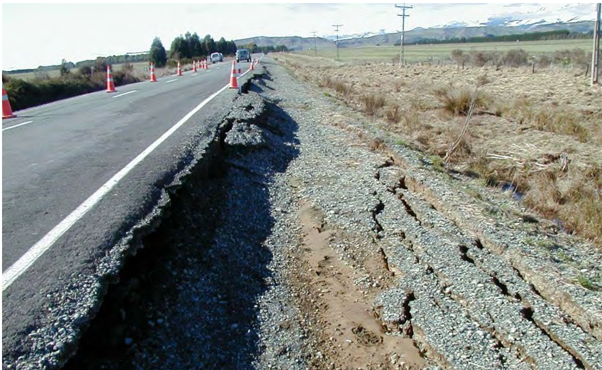
Figure 8 Damage to Hillside Road, Manapouri, Southland, resulting from the 2003 Fiordland earthquake. The road is raised on an embankment. Disaggregation of the embankment fill by ground shaking has caused a lateral spreading failure of the margins of the embankment. The existence of the embankment reflects the soft and saturated nature of the ground here, which probably exacerbated the earthquake shaking and consequential damage to the road. Photo: R Cook.
